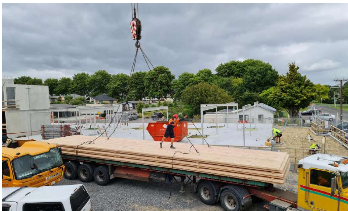
Figure 27: Site safety officer is checking all equipment and components related to the lifting process.
