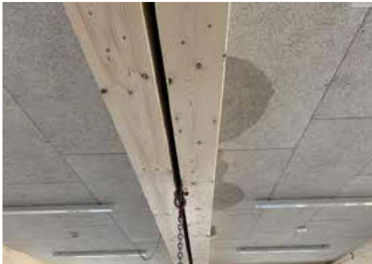
Figure 31: Leaking joint in mass timber [2] .
