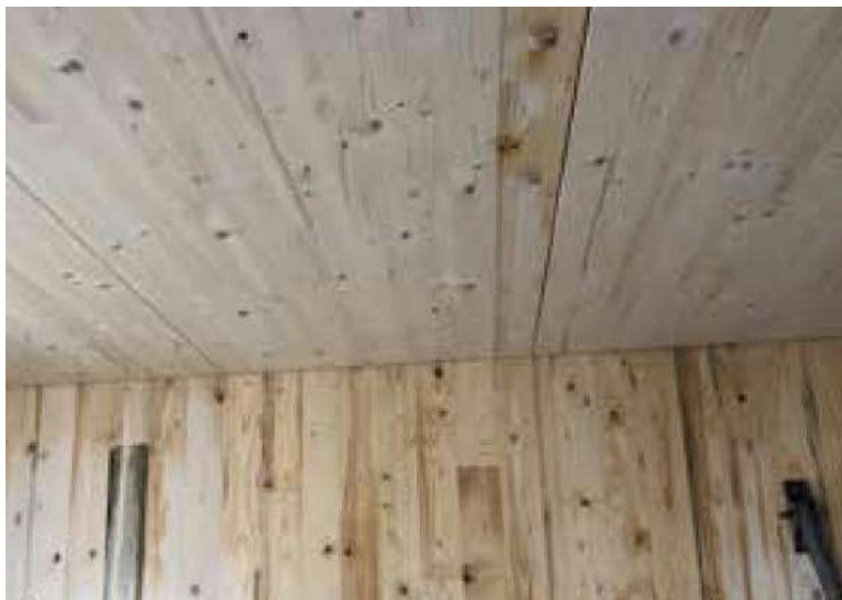
Figure 29: Stains due to water ingress [2] .
