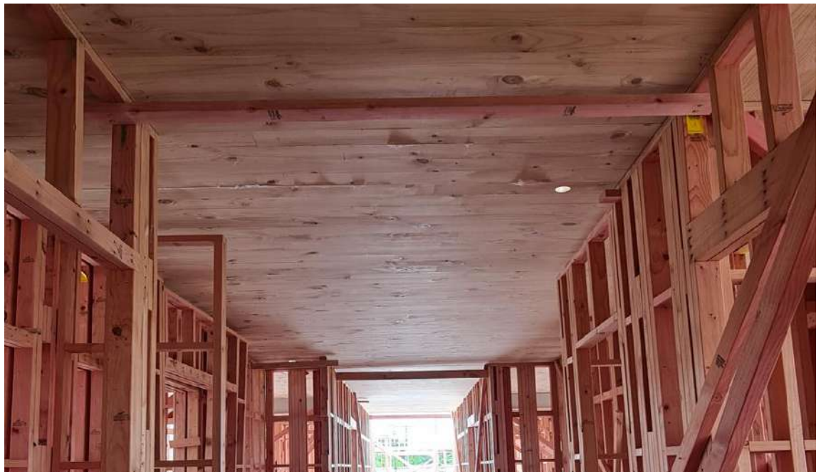
Figure 18: Red Stag CLT midfloor over the Red Stag light timber framing (Red Stag has a frame and truss manufacturing plant in Hamilton, New Zealand that can integrate supply into a hybrid mass and light timber project).
