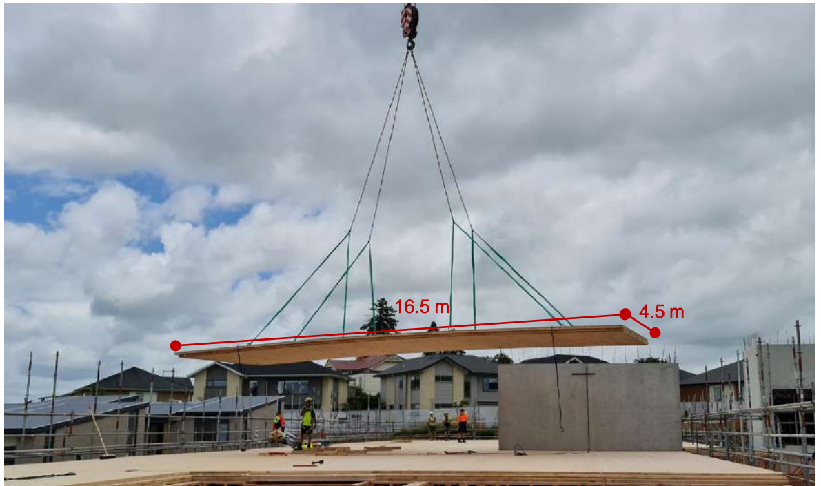
Figure 17: Installation shows an example of a 75 square meter Red Stag CLT panel being effortlessly installed on site. 16.5 m x 4.5 m Red Stag CLT floor panel is lifted via eight screw anchor lifting points.
