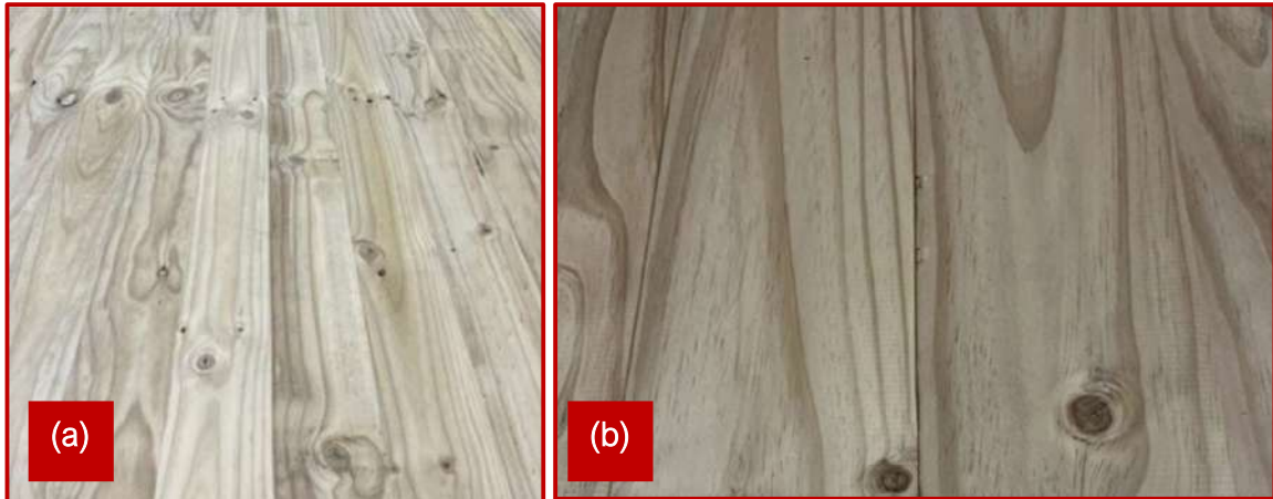
Figure 146: Red Stag H3.2 treated EWP panels generating a slight green tinge; a) Open View; b) Close View.
