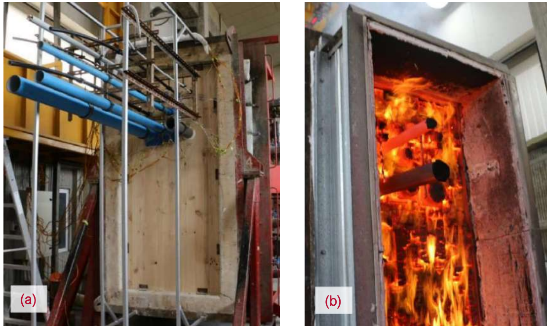
Figure 75: Various service (pipes and cables) fire tests on Red Stag CLT wall panels [26] . a) Specimen before the fire test, b) Specimen after the fire test.
