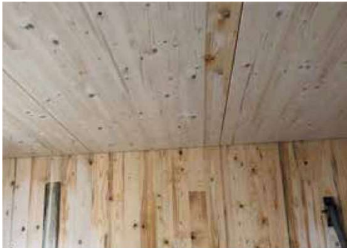
Figure 29: Stains due to water ingress [2] .
