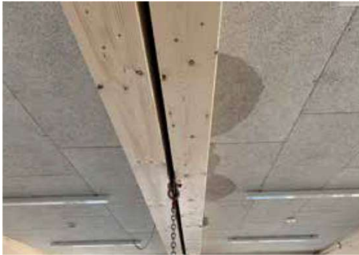
Figure 31: Leaking joint in mass timber [2] .
