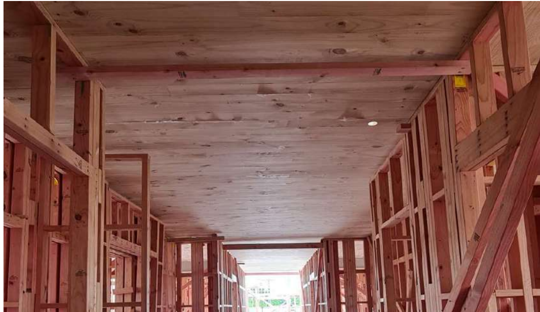
Figure 18: Red Stag CLT midfloor over the Red Stag light timber framing (Red Stag has a frame and truss manufacturing plant in Hamilton, New Zealand that can integrate supply into a hybrid mass and light timber projects).
